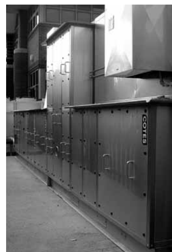
Installing the Cotes dehumidification system at the Nexeon facility.
